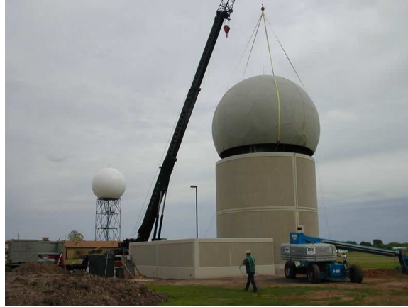
Figure 1: Photograph of the NWRT PAR system during radome installation. The antenna array is housed inside the dome at approximately 12 m above the ground.
