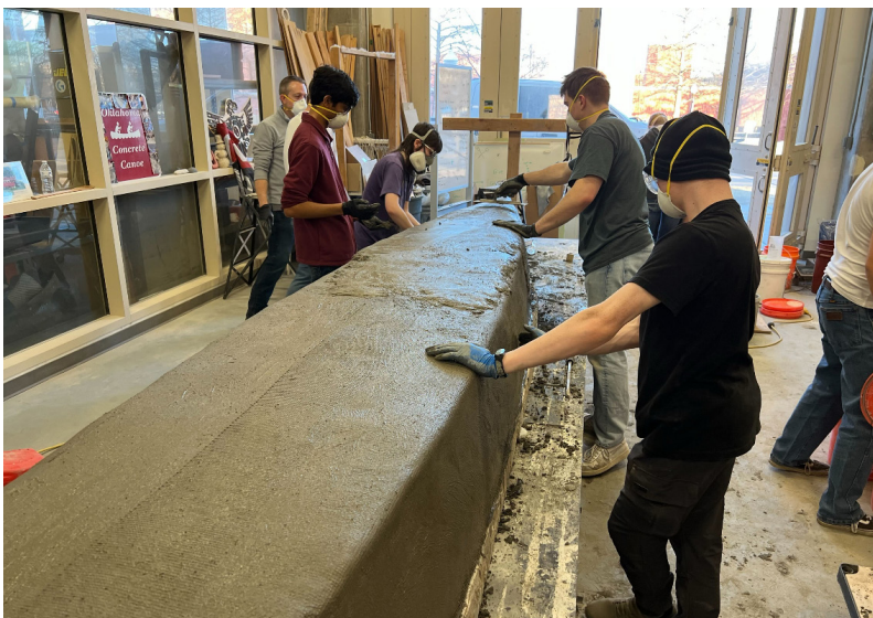
The Concrete Canoe team fabricating its vessel in the Engineering Practice Facility. This student competition group designs, constructs, and tests a canoe made entirely of concrete that is strong enough to support student rowers.
